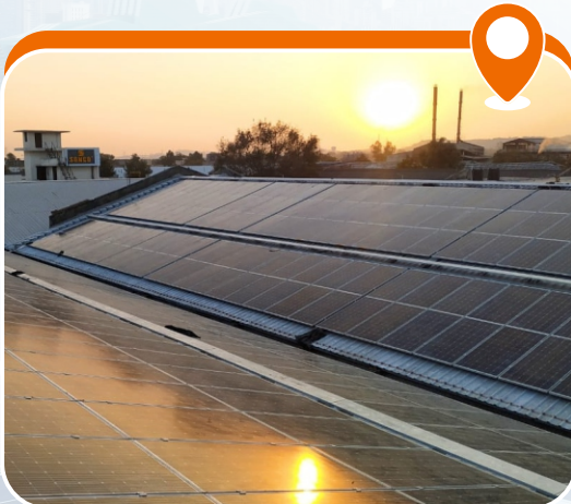
210 KW Pinaka Power
