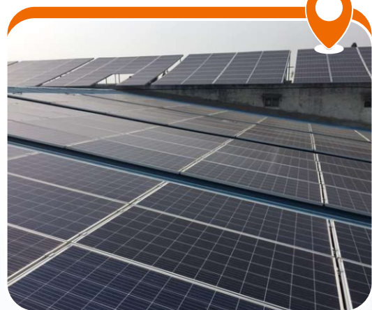
85 KW Kamal Glass Solution Pvt Ltd.
