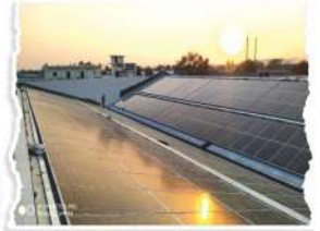
210 KW Pinaka Power
