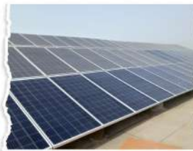
65 KW Patel Hospital
